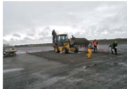
Raking out and compacting the base material to provide a solid, well drained foundation for the Endura-Form installation
