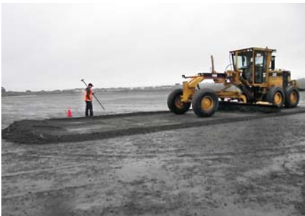
We started site preparation to provide a firm foundation for the Endura-Form Panel installation.
