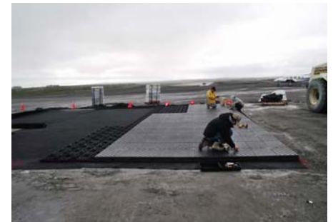
The layout of the Endura-Form panels starts over top a layer of material.
